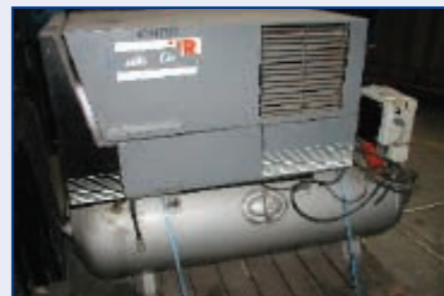
Schroefcompressor/Screw-type compressor ATLAS COPCO, type Hydrovan 120.
