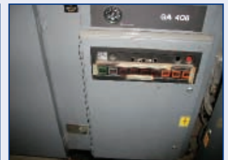
2 st. Compressoren/2 off Compressors ATLAS COPCO, type GA 408, cap. 8 bar.
