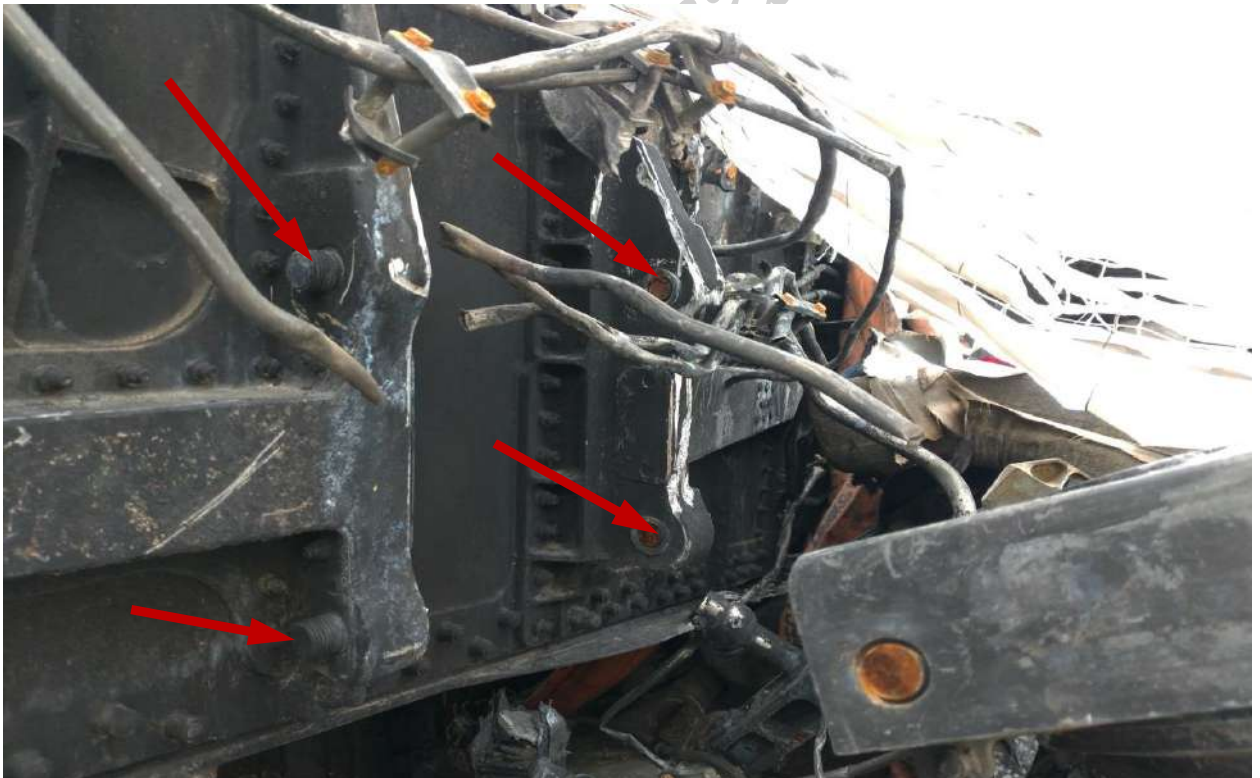
Fig. 19. The right MLG attachment A fitting on the rear spar adjacent to rib 3, the attachment A fuse pins («weak links») are sheared
