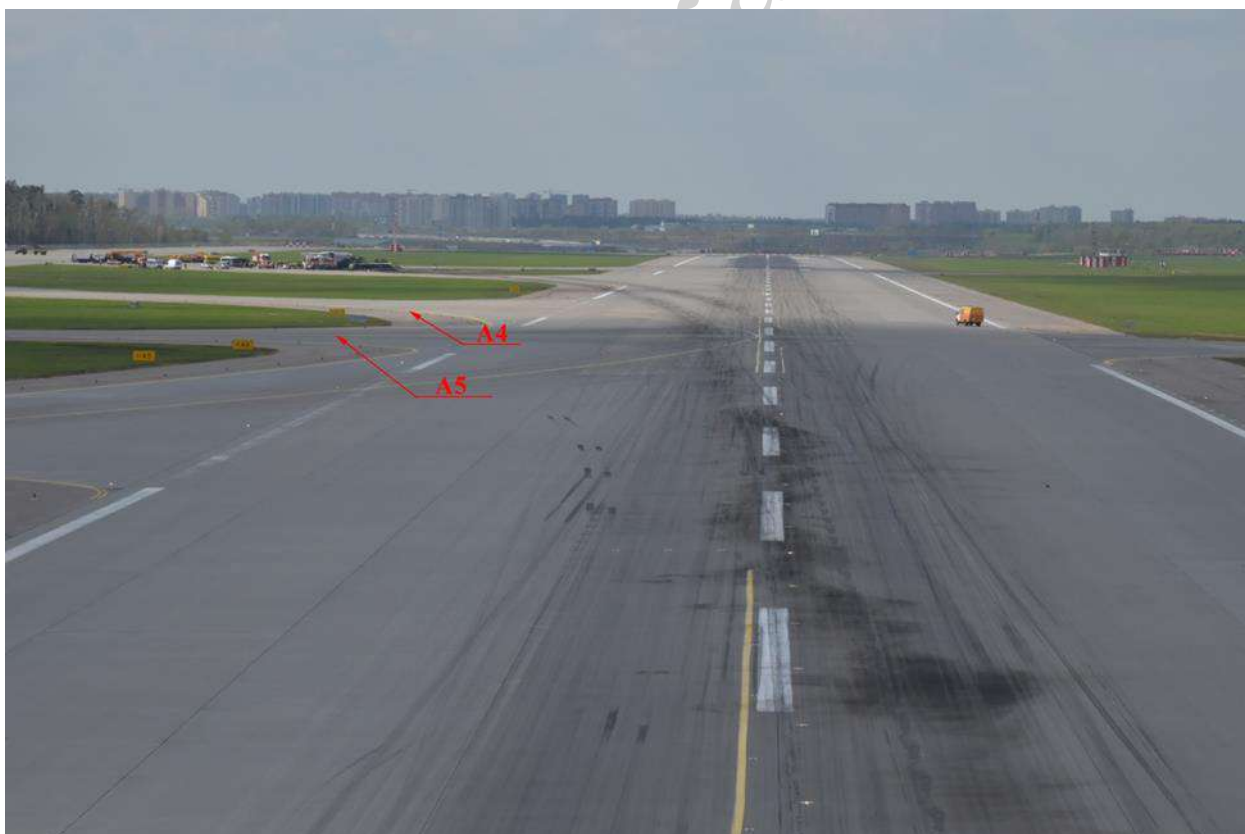
Fig. 38. The starting point of the traces shift to the left off the RWY centerline at the area of the A5 TWY
