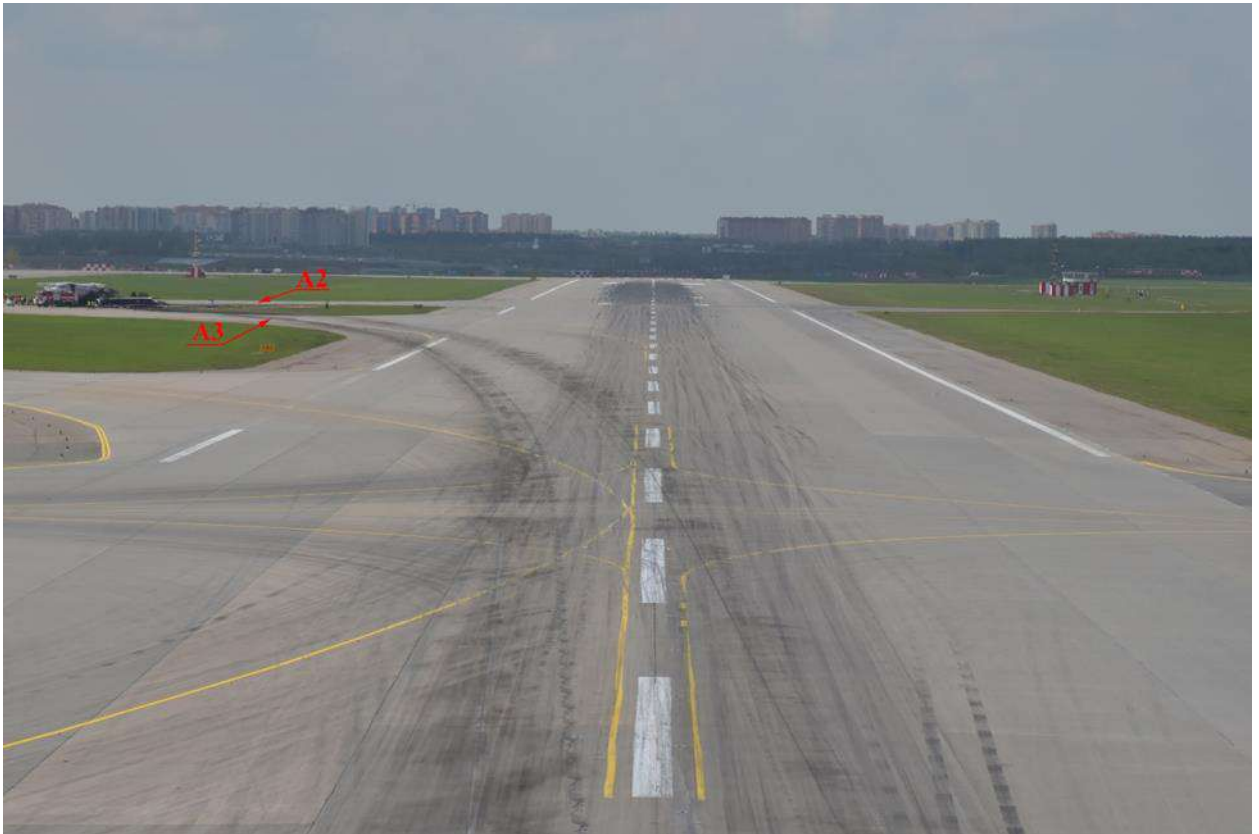
Fig. 39. The traces of the aircraft movement, the spot of the veering off the RWY at the area of the A3 TWY
