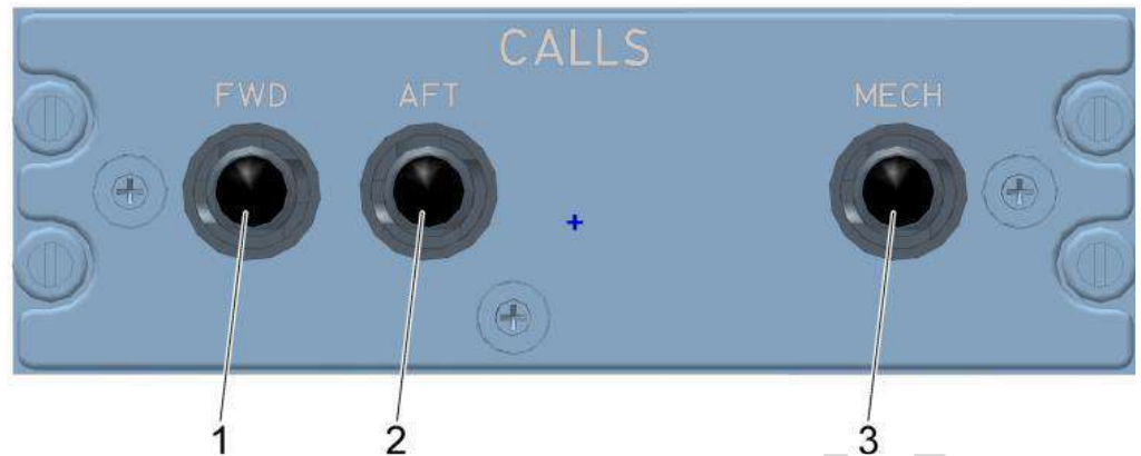
Fig. 136. The exterior of the individual calls control panel
